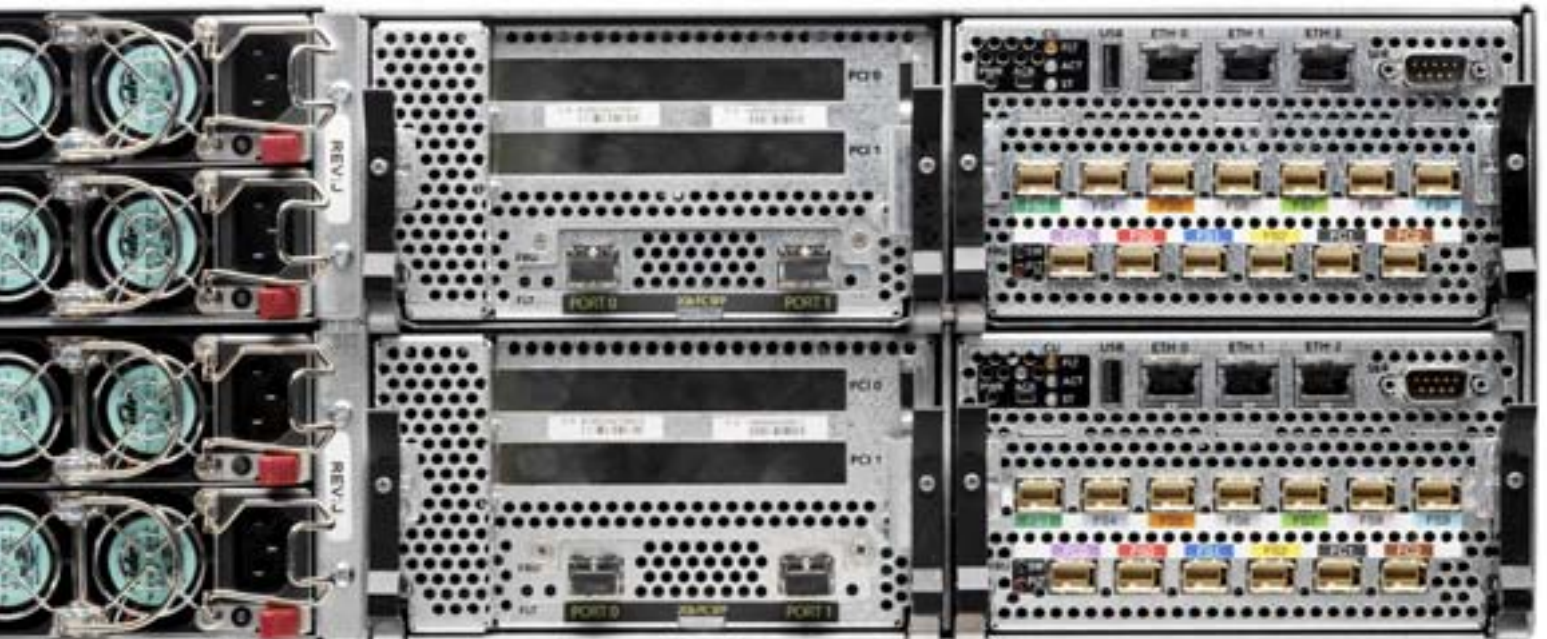
Rear View of the Pillar Axiom Slammer Storage Controller
